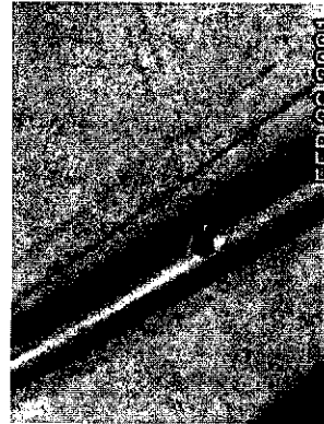
Photo: Lower rib location 1/2" hole, rear of spar.
